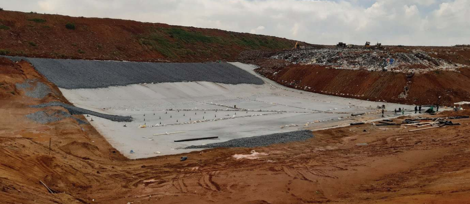
The Waste Group Class B liner being completed at the Mooiplaas landfill site in Centurion, Gauteng
